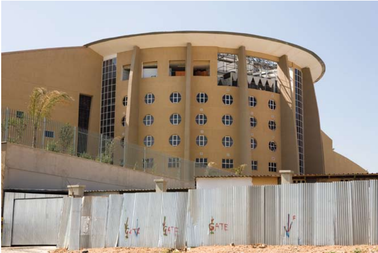
The Universal Church of the Kingdom of God nearing completion in Diepkloof, Soweto.
